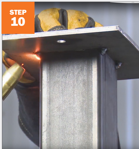
STEP 10 Double check for square, then finish welding the top plate to the post.
