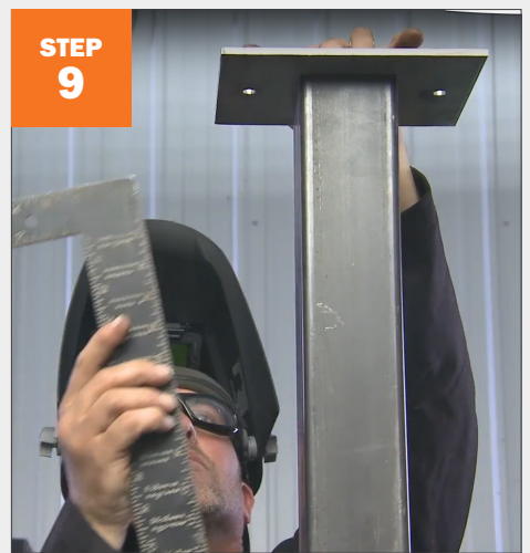
STEP 9 Make sure post and top plate are square, then tack weld into place.
